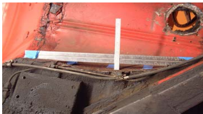
Fig 7 Here's the after shot. Bend the sheetmetal clamp over the fuel line.
