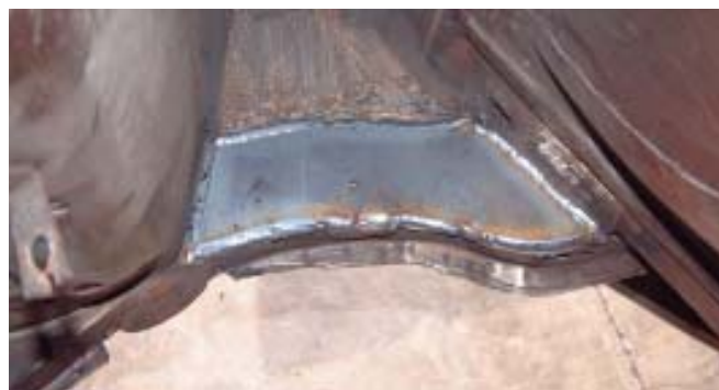
Figure 7. This is how the completely welded perimeter plate should appear when you're done welding. You can grind these edges smooth if you like, or simply notch the 3/16 front piece to fit the weld buildup as required.
