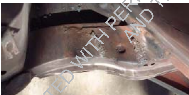
Figure 4. Here's a shot of what you'd have if you removed the OEM Panhard frame bracket before it fails. This is as close as you want to get with a cutting torch. The rest must be ground down to the frame surface.
