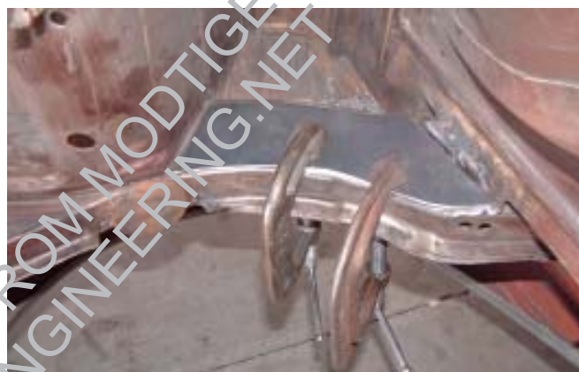
Figure 6. Here we have the cover plate placed and clamped to the frame. You're going to want to even out the gap at the perimeter so that you can weld to the edge of the frame in the area of the bends. This will give you the strongest attachment.
