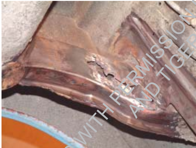
Figure 1. Here we have a fairly typical frame failure where the U shaped mount has torn loose from the frame and has taken a substantial portion of the side of the frame with it. This is another area where repeated stress has fatigued the sheetmetal frame. This is not normally an area that is subject to rust, so it's simply been overworked.
