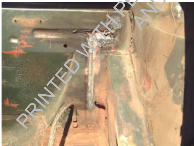
Figure 14. Here's a shot of the trunk showing the substantial weld penetration in the back wall of the trunk. In all cases, this will require a repainting of this area, but this is a small price to pay for the increased durability of this installation.
