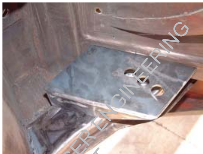
Figure 10. Here we have the mount placed and aligned with both the side plate on the frame and the stamped bump in the back wall of the trunk.
